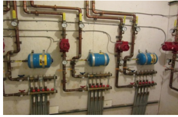
Geothermal Heat Pump System – Sikh Temple Virginia
